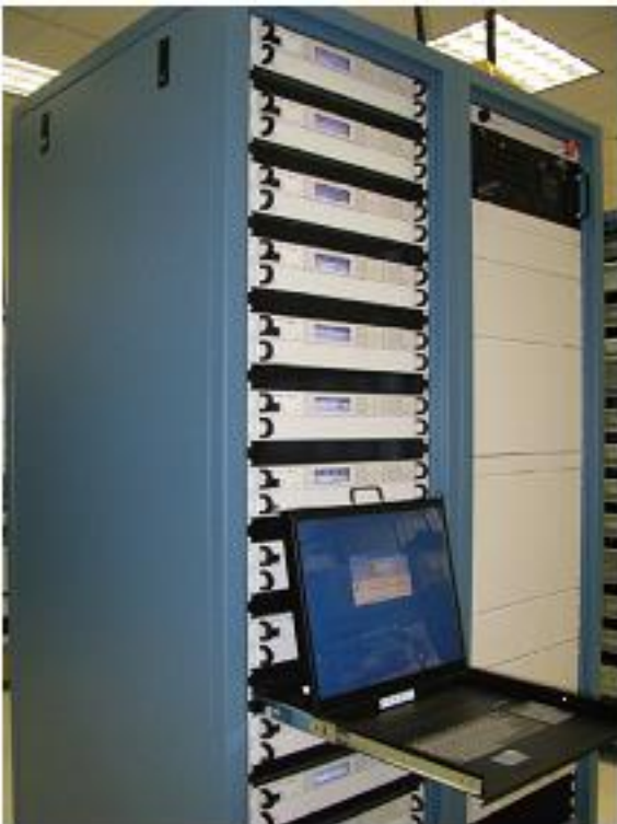
Figure 7.14 – This rack uses 12 Keysight E4360A units to supply 24 channels for simulation.
